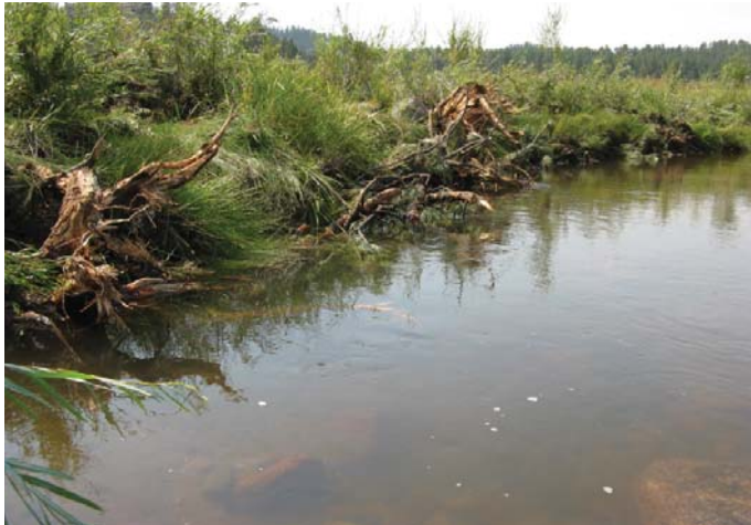
top: Eroding bank typical of pre-restoration conditions bottom: Stream bank following restoration
