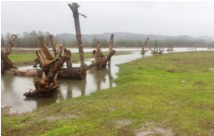
top: Newly daylighted channels and vegetated mats before riparian planting above: Newly installed large wood
