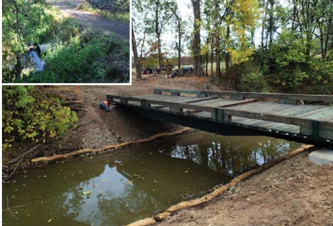
The replacement of an undersized culvert with a refurbished rail car bridge provides fish passage and hydraulic connectivity; inset: initial conditions
