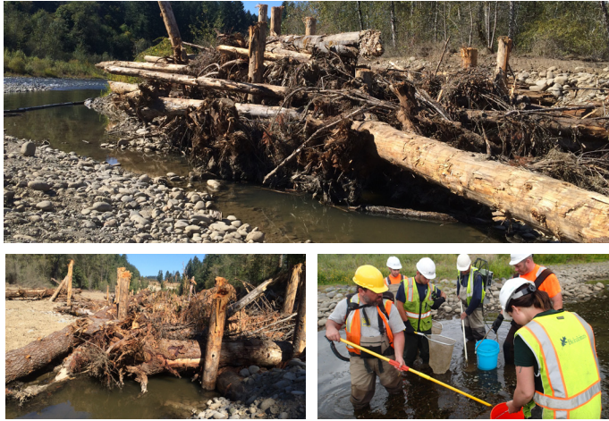
clockwise from top: The renewed Goose Creek confluence; The team quickly removes biota from work area; Log installations provide shelter for many species
