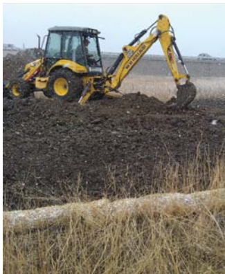
from top: Timberline wetland one year after restoration; I-25/392 wetland during construction
