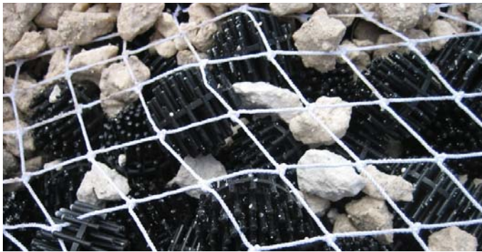
from top: Subsurface flow constructed wetland immediately after planting; Bioballs and gravel wetland treatment media
