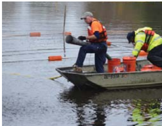
from top: Tidal wetland bench (left background) immediately after planting; Installation of sand utilizing a Telebelt®; Placement of SediMite™ from a boat using compressed air
