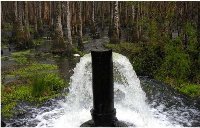
from top: Constructed wetland with trickling filters; Treated effluent used for land application in a cypress forest
