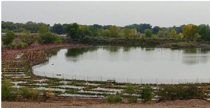
From top: Kingfisher Gadwall Pond before construction can be seen with steep banks, old gravel, and no wetland edges; Kingfisher Gadwall Pond after construction, now with wide wetland benches, sod mats created from local wetland vegetation seed, and a transition to uplands.
