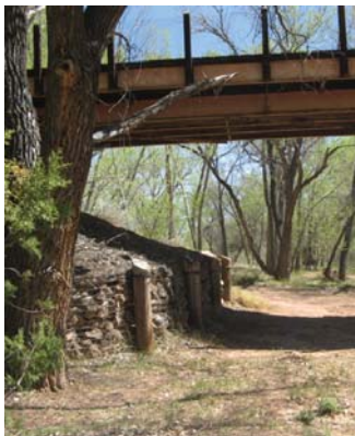
from top: Post vane structure with willow plantings; Historic "El Puente" wooden bridge over Galisteo Creek
