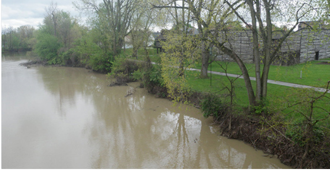
Erosion in front of old fort along the Saint Mary's River
