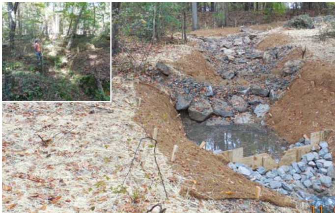
Upstream (top) and downstream (above) immediately after construction with initial conditions inset
