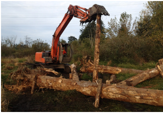
from top: Restoration mitigates flooding impacts and improves habitat and water quality; Assessing options for installation of large wood; Installing large wood under challenging conditions
