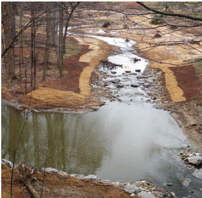
clockwise from top left: Detail of conceptual design; Installing a boulder riffle; Immediately after construction
